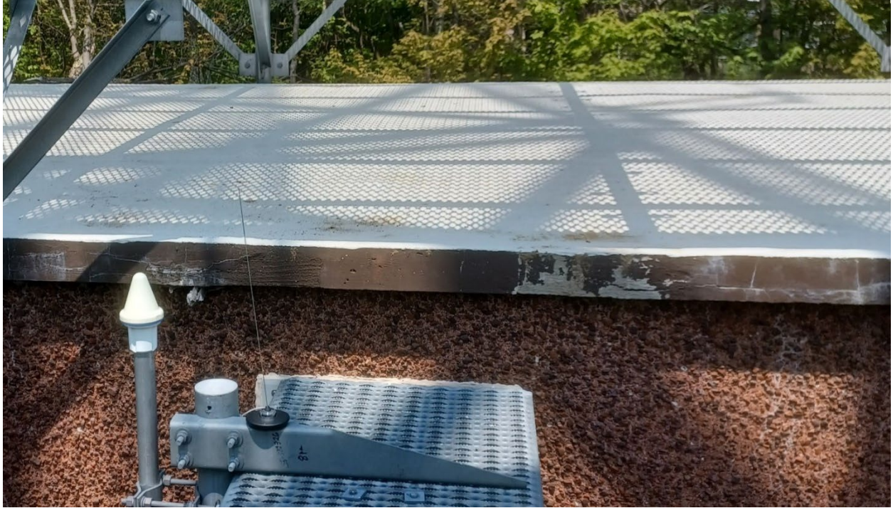
Area most likely responsible for water entry
